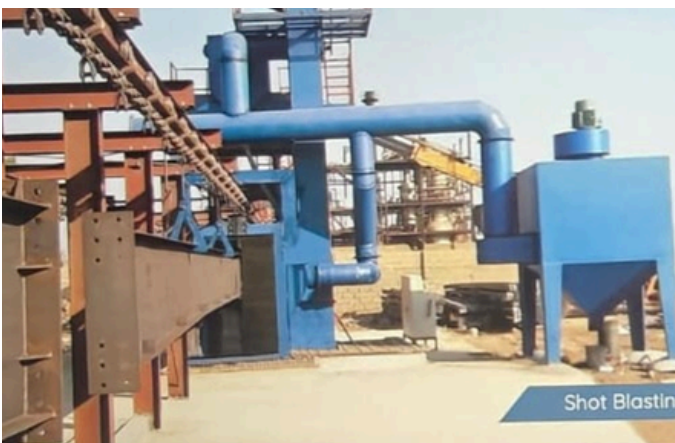
Blasting & Painting Facility
